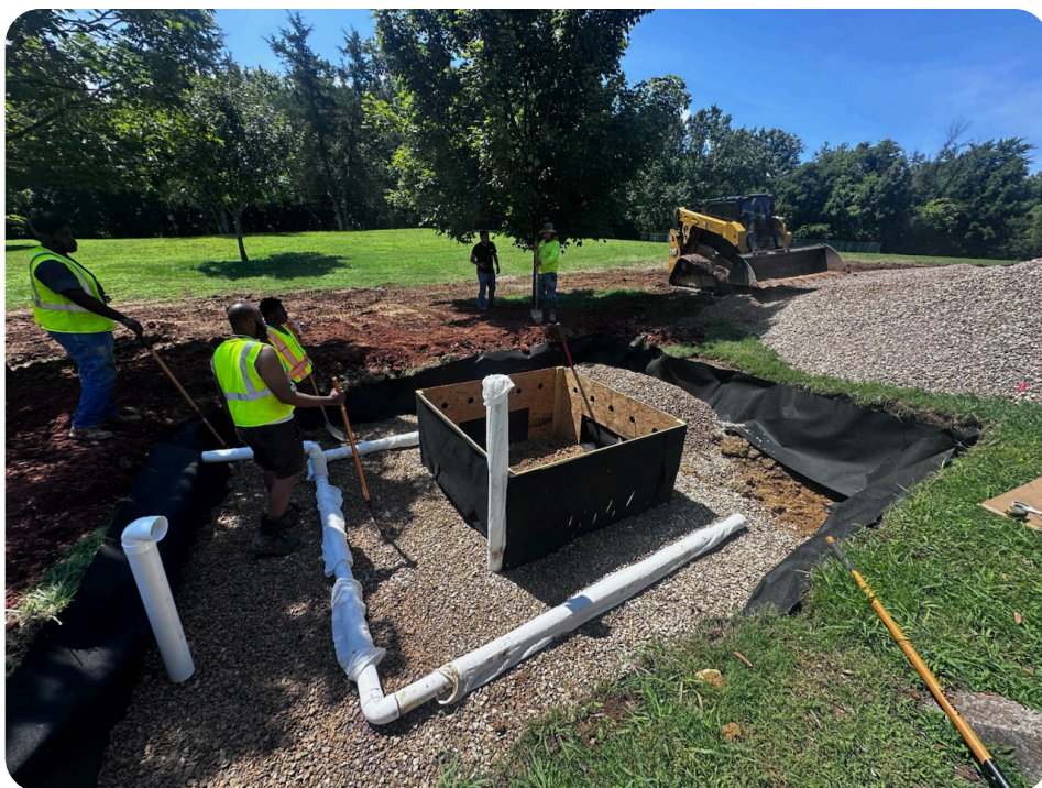
The installation of a GTSS - this is what's going on underneath the gravel. The box in the center will be filled with soil and have a tree planted on top, and the PVC pipe with holes around the box will be buried under gravel.
